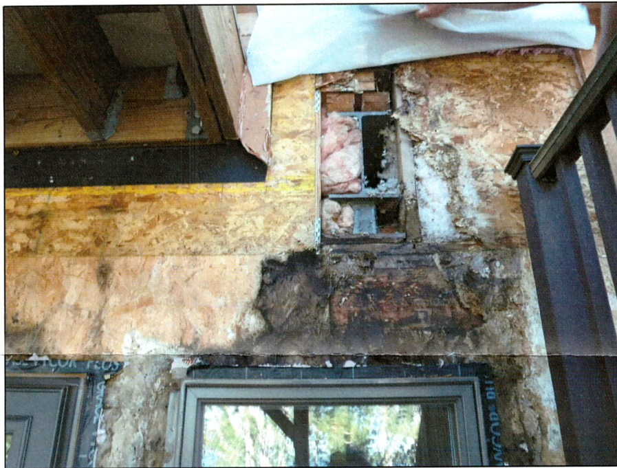
Steel Beam Bearing On Rotted Header
