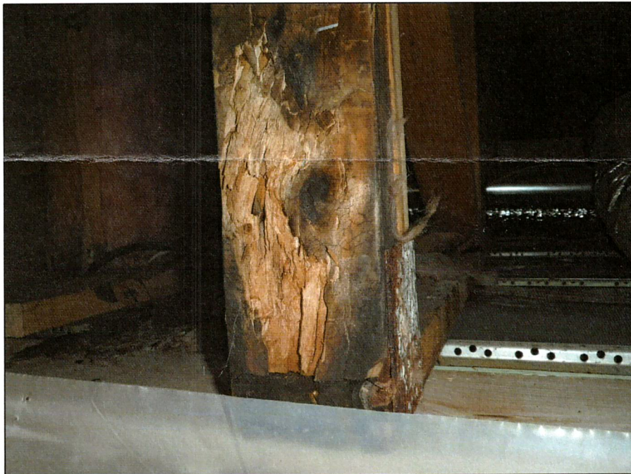
Rotted Floor Truss
